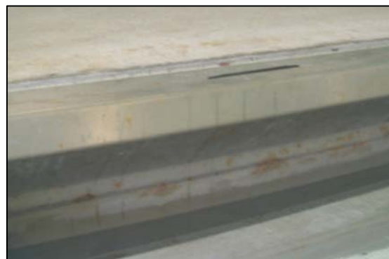
Fig 5. Corrosion in trough
