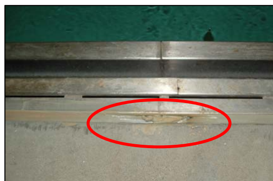
Fig 6. Gap in sealant
